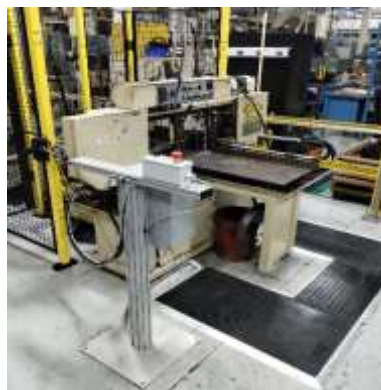
Horizontal bandsaw (lg) guard with safety mat and remote controls
